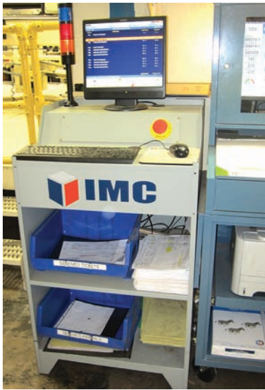
A Pacesetter control system from Intelligent Machine Control, was among the retrofits.
